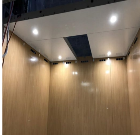
Gayhead's new elevator
